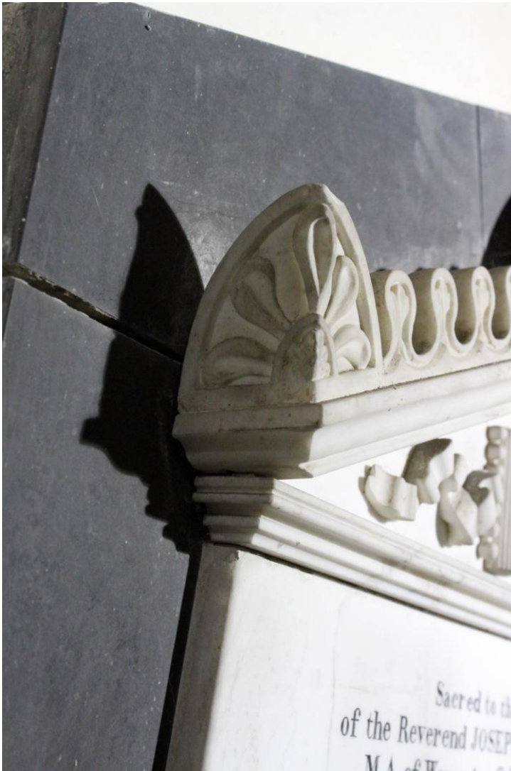
Above: open joints in the structure, caused by corrosion of fixings
