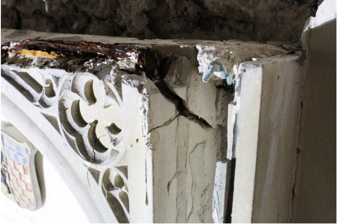
Top photo: dismantling in progress, showing large iron clamp; below, fractured stones laid out before repair
